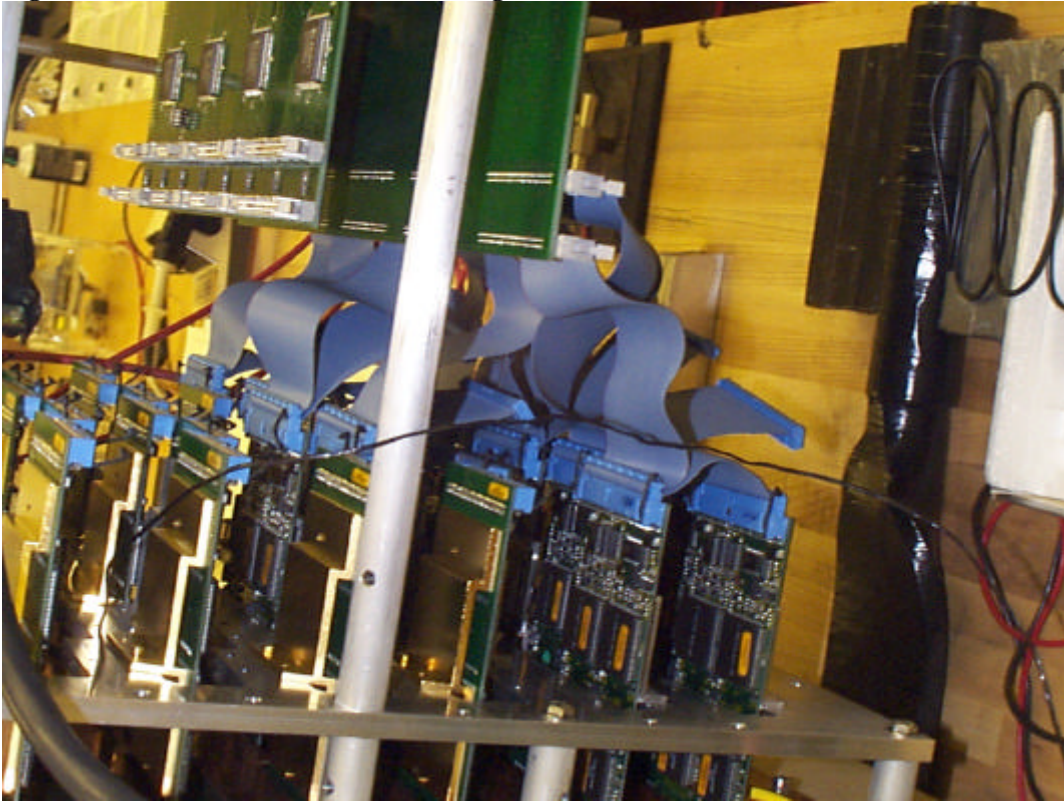
Fig.4 Side view of MTP1. Before cabling of aux. Board.
